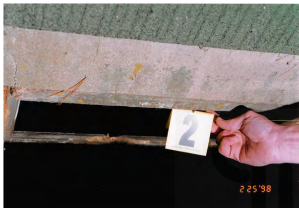
Figure 26 - BCA crime scene photograph of south window well
